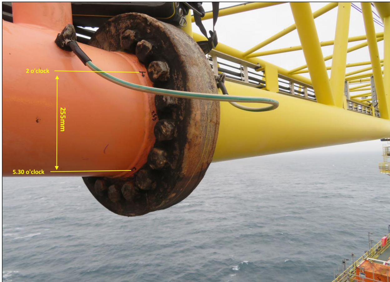
Photo shows location of the manufacturing defect found on Chord D flange connection weld measuring 255mm.
