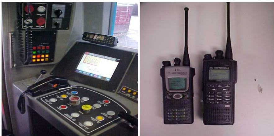
FIGURE 9.1: TRAIN CAB RADIO AND COMM. FACILITY FOR MAINTENANCE
