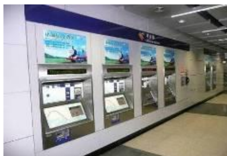
MTR Wall mounted TVM with maintenance corridor in the back – Paris
